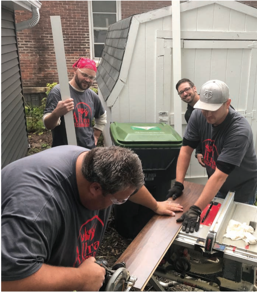
Members of the mortgage department at Altra CU work on a Habitat for Humanity home on Altra Gives Back Day.
